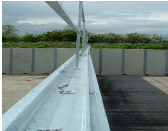
Photograph 2: Channel to guide retractable roof and rainwater
