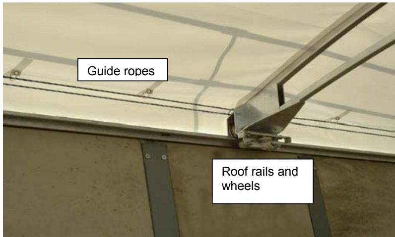
Photograph 4: Roof rails guided by wheels and moved back and fro using ropes
